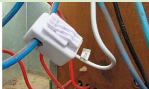
1 The Clip-On Sensor simply attaches to the main active or phase cable at the switchboard.
