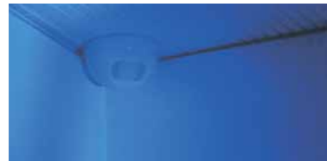
Automatically turn lights off with a sensor.
